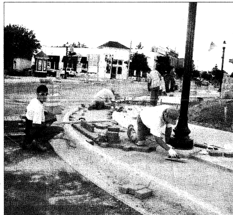
The Boyne City sidewalks in some areas downtown are being reconstructed with bricks. Working on the sidewalks in the foreground are Lance Pankratz (left) and Tom Haley of Haley Construction Company.
