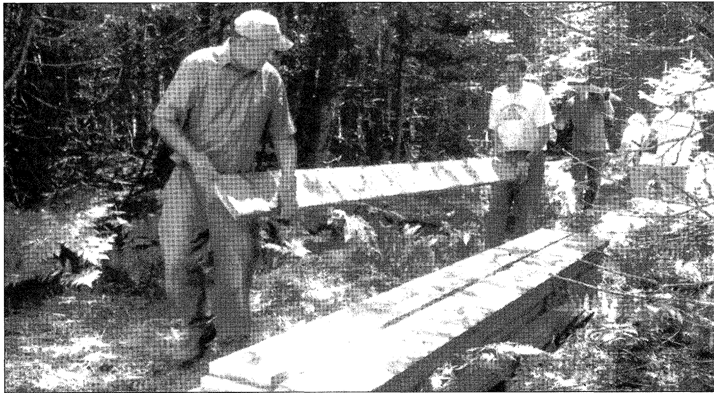
Volunteers haul lumber to build the boardwalk connecting Susan Creek and Taimi Hoag Nature Preserves.
