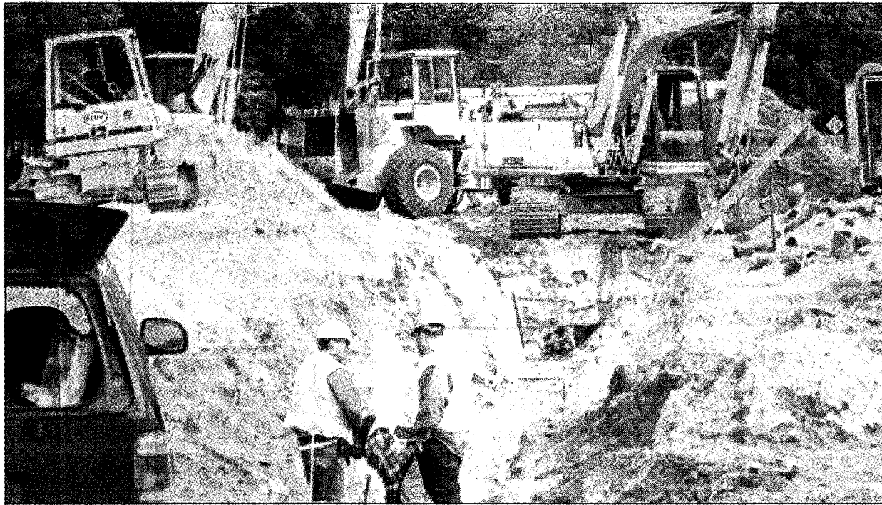
Boyne City's State Street, between Park and North East, transformed from a big hole in the ground as shown, to a nearly paveable surface just a day later.
