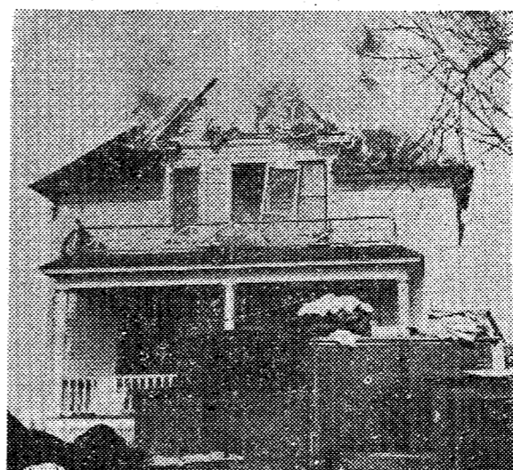
They did not replace electric cords that had frayed ...
