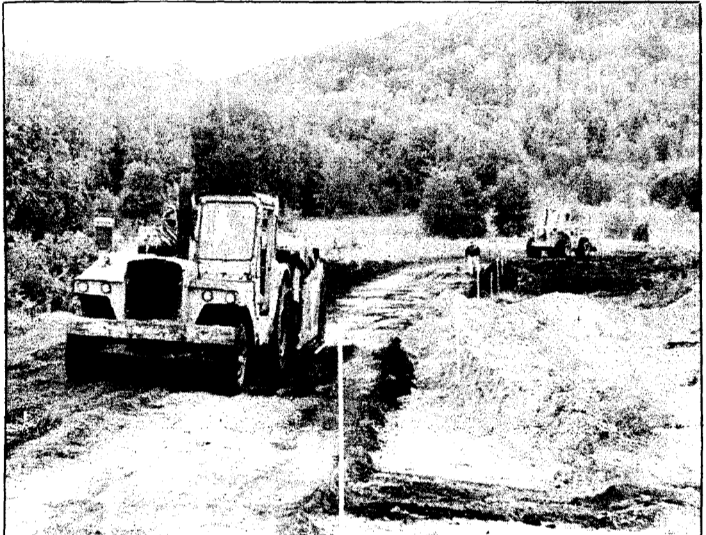
The beginning of the building boom took off this past week in Boyne City as ground was broken and site work started for a 24 unit apartment project on Division Street. The project, headed up by Scott Dietze and Richard Brooks, will feature apartments for singles and families. Other projects set to get underway around Boyne City include the expansion of the runway at the airport, installation of sewer and water lines to the Air-Industrial Park, the Peninsula Beach project, and the building of the LexaMar plant in the industrial park.
