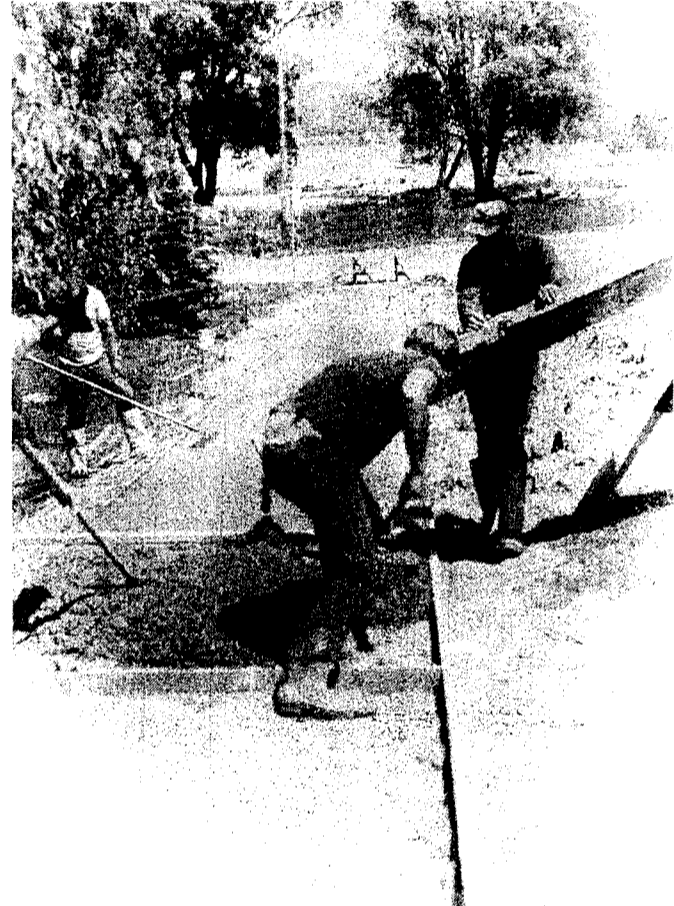
Boyerne City has a new bit of sidewalk as city and O.D. Sayles crews worked last week to lay this block long piece of cement along Pleasant Avenue. The sidewalk required filling the ground around it to keep the walk at the same level as the road.
