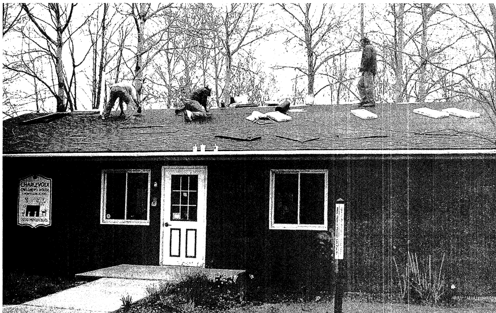
Ron Schroeder Construction crew members, Tim, Corey and Ron Schroeder, donated their labor for installing a new roof on the Charlevoix Children's House in mid April. COURTESY PHOTO
