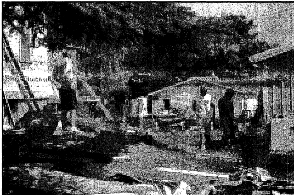
A full crew, including nearly a dozen high school students, showed up at the Doty house on Saturday, June 27, ready to re-side.
