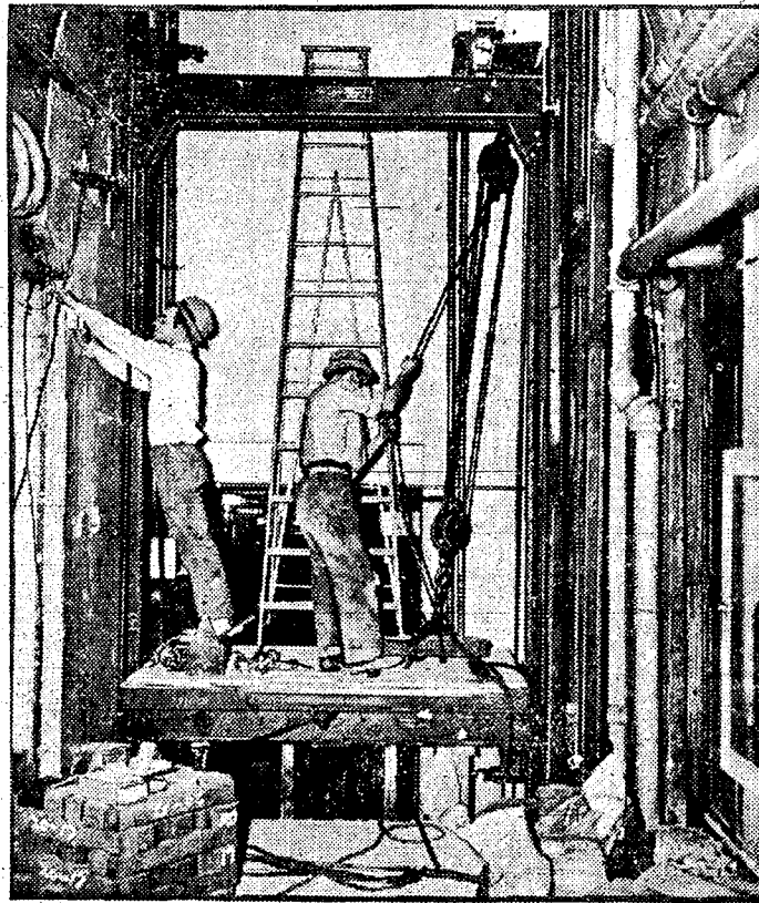
Workmen are shown installing new high-speed elevators in the Capitol building in Washington. The old ones were too slow for the congressmen.
