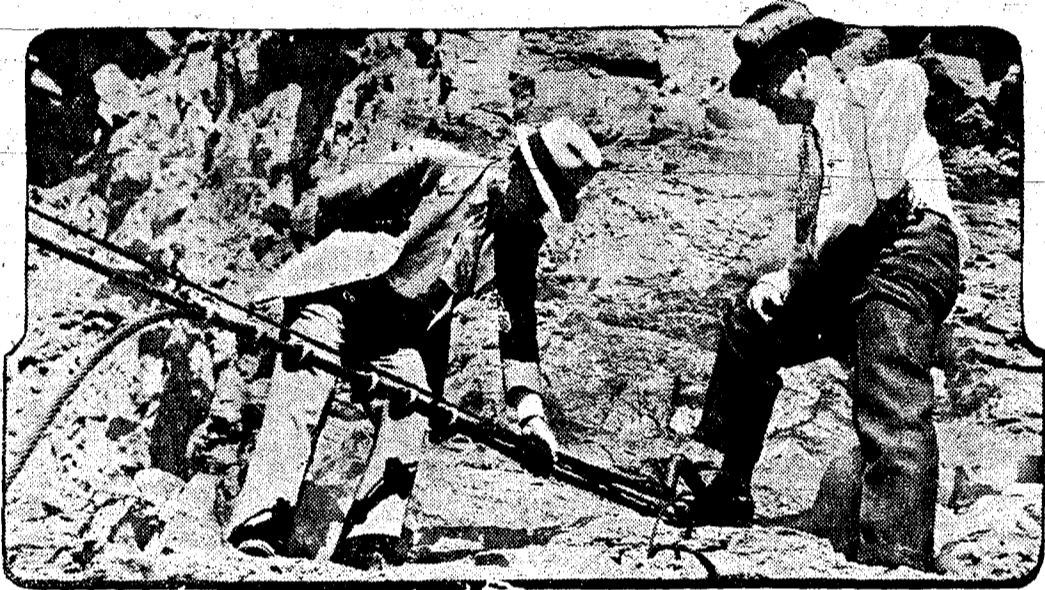
Major F. L. Pomeroy of the Arizona National Guard announced that Arizona's rights had been encroached upon through the anchoring of several cables in Arizona territory in the sensational state squabble over construction of the Parker diversion dam by the metropolitan water district of southern California. Arizona National Guardsmen were sent to the dam site to protect the state's rights. Pictured here, left to right, are Major Pomeroy and Herbert H. Hotchkiss, secretary to Governor Moeur, examining a cable anchored in Arizona territory.
