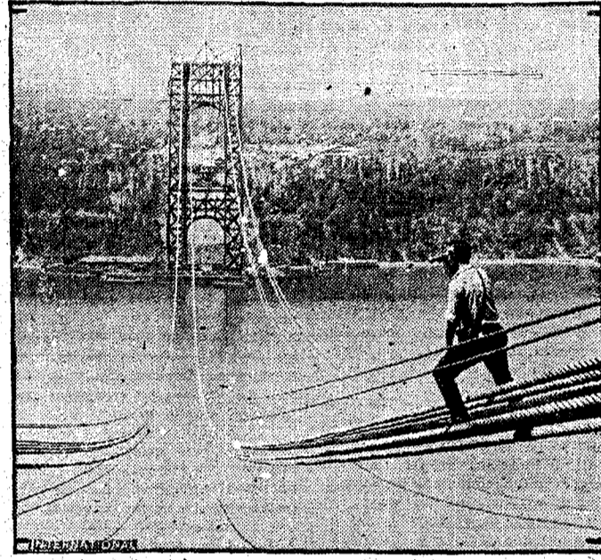
A. M. Nelson, instructor of engineering at West Point, risking his life during inspection of foot bridge cable adjustment for the Hudson river bridge, that will be longest suspension span in the world. The slightest slip would have sent Nelson hurtling hundreds of feet below to the Hudson river.
